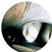
Valves: Check condition without dismantling
